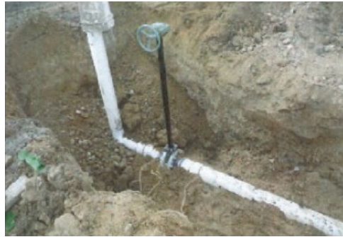
Figure 3 Discharge Well Setup for the Pilot Mitigation Program. The Valve Seen in the Figure Allowed for the Controlled Release of Artesian Groundwater at Various Rates
