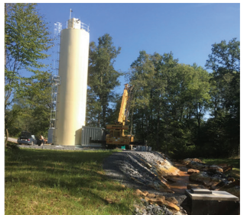
Figure 5 Glade Run doser with in-stream pH probe in the foreground right (image: Chester Wright, OSR)
