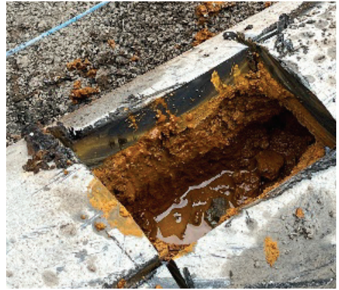
Figure 8 Iron accumulation in AMD pressurized line (image: Greg Phillips)
