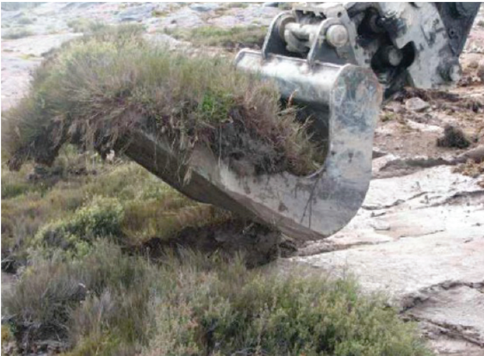
Figure 1 Specialised VDT stripping head reverse-attached to an excavator bucket. Photo by D Rodgers.
