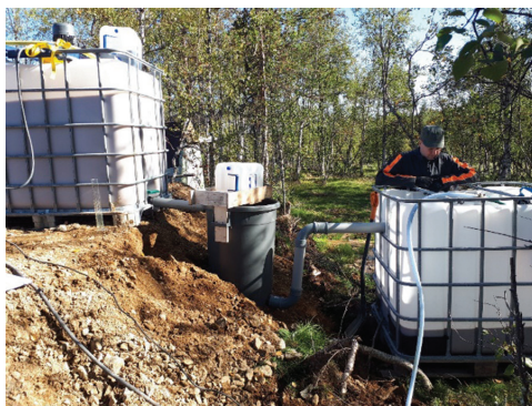
Figure 2 Ongoing field tests, left IBC on dam of circulation pond. (photo: E. Takaluoma).
