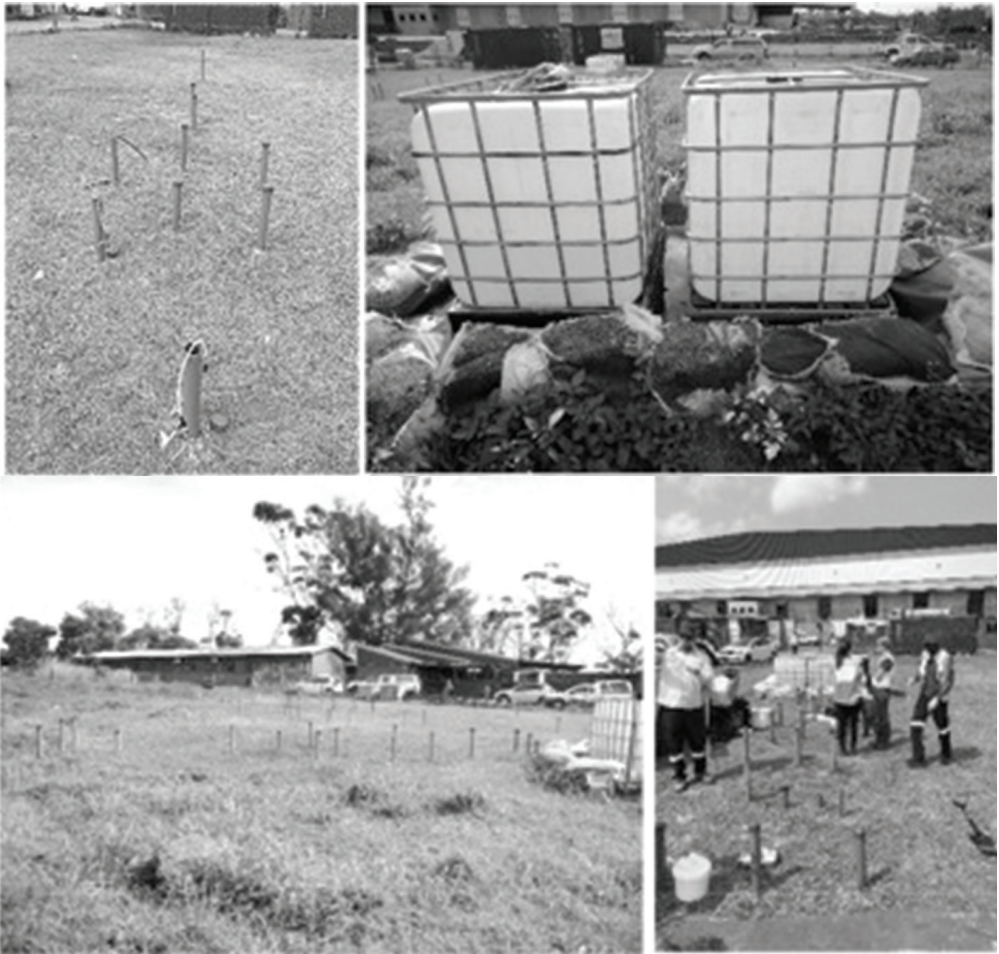
Figure 1 In situ treatment implemented at site A, located in the KwaZulu Natal province of South Africa.
