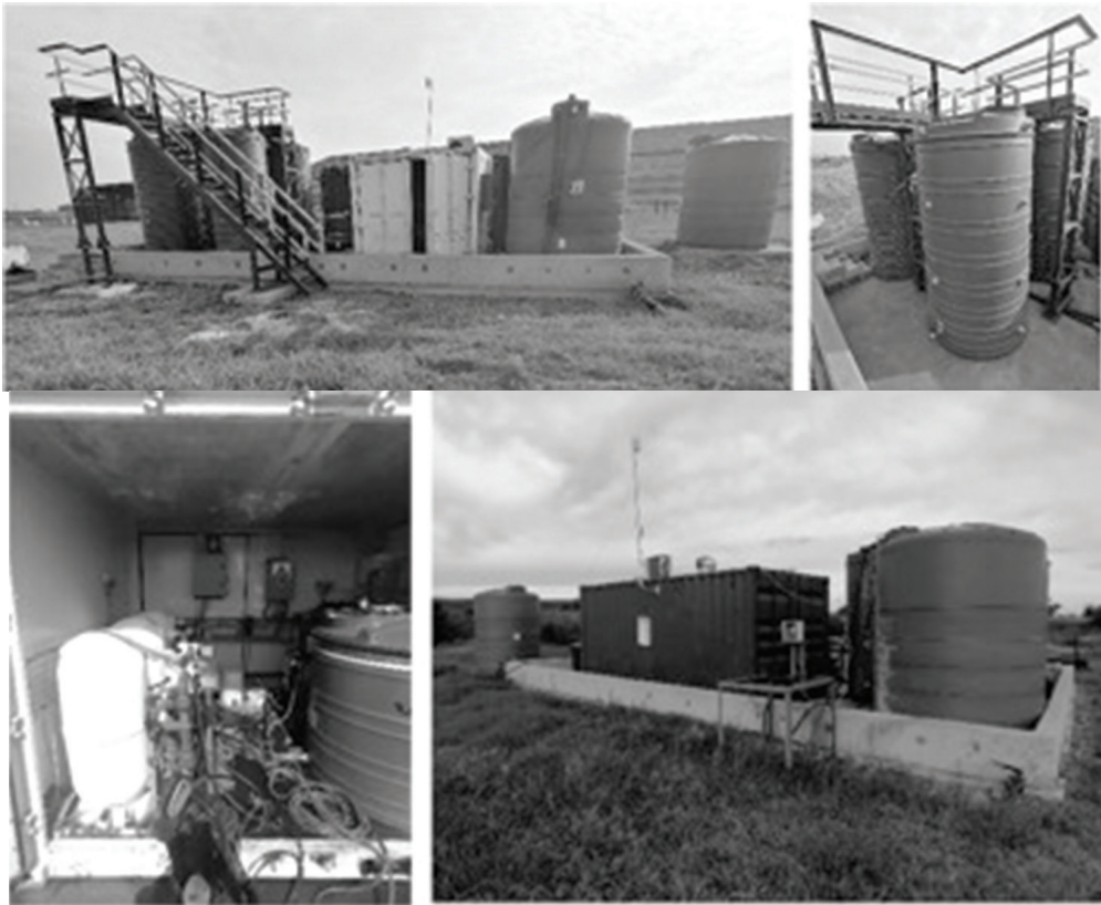
Figure 2 Semi-active pump and treat plant implemented at site B, located in the North West province of South Africa.
