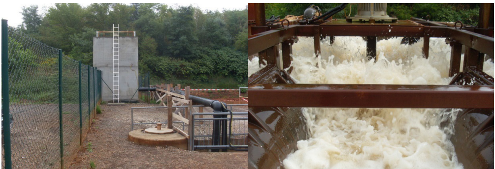
Figure 1 View on the pre-aeration tank (left side) and the surface aerator in operation (right side).
