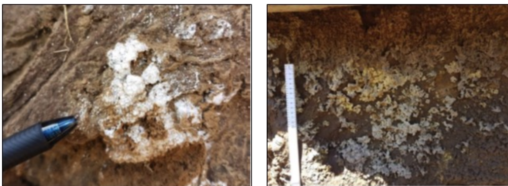
Figure 2 A) Efflorescent crusts on the sidewalls of the Glynn's Lydenburg TSF. B) Efflorescent crust developed on the slopes of the Nestor TSF
