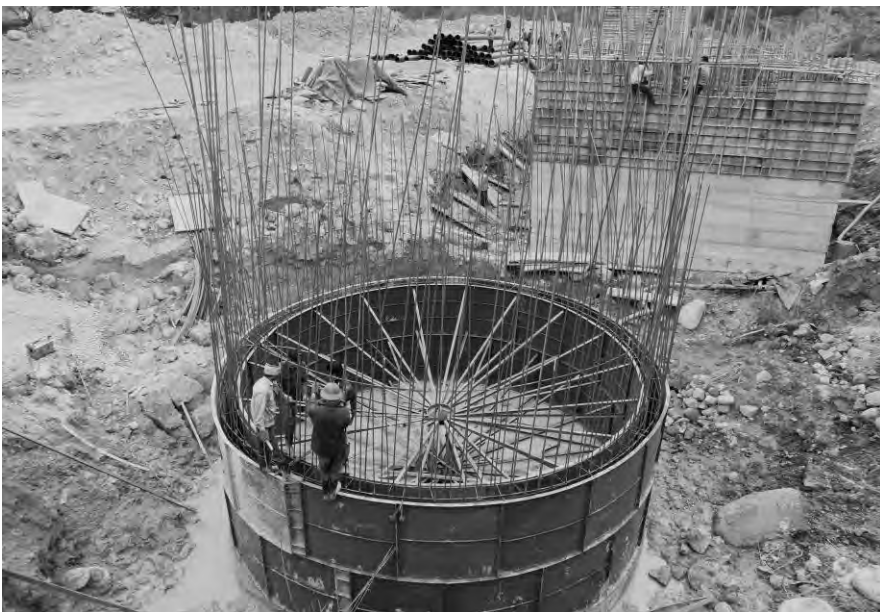
Figure 4 Erection of the sludge thickener in Vang Danh (sedimentation basin in the background).
