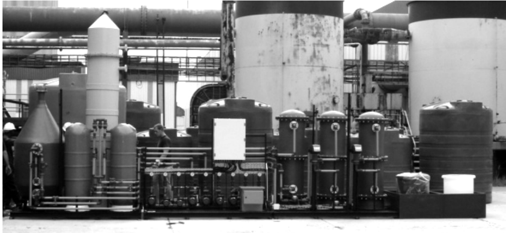
Figure 6. Mine Process Water Pilot Plant
