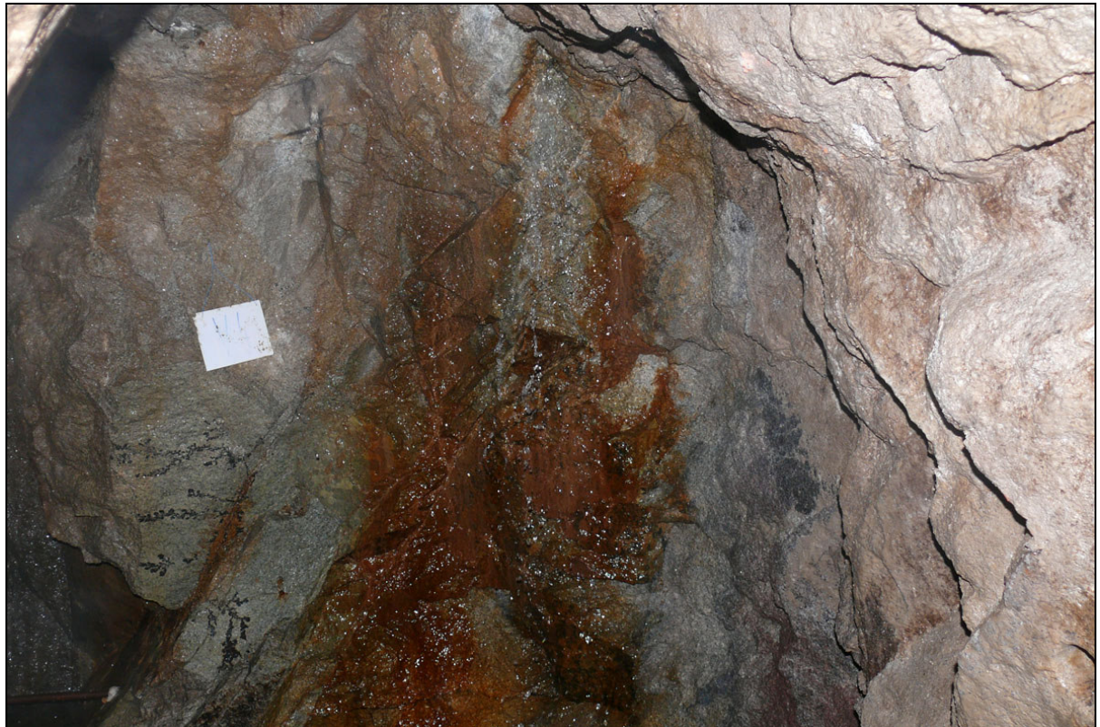
Supplement 2 Running water from crack
