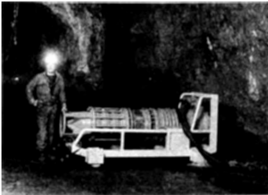
Fig. 2. HEAVY DUTY HIGH HEAD SUBMERSIBLE MAIN DEWATERING PUMP PLACED ON A SKID.
